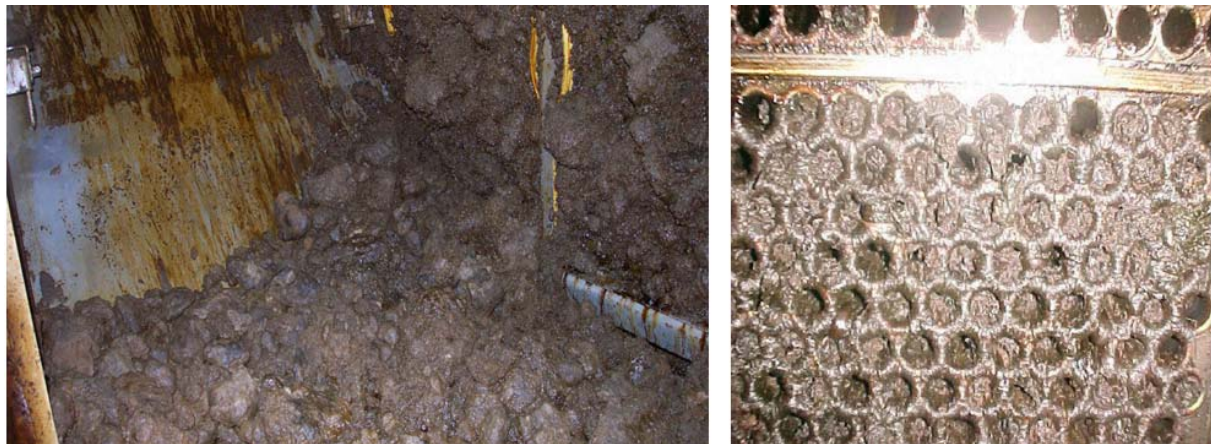
Figure 2.5 Naphthenate deposit in separator (left)[46] and in process heater (right)[47]
