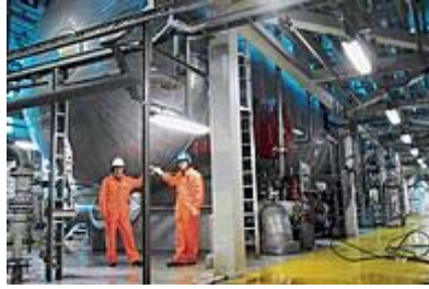
Figure 4-6 First stage separator tank with VIEC installed. 82
