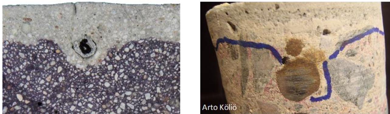
Figure 12: Left: cross section of reinforced mortar sample (6-mm rebar) sprayed with thymolphthalein [Belda Revert et al., In preparation]. Right: reinforced concrete core sprayed with phenolphthalein (fading), uneven carbonation front indicated by blue line. Courtesy of A. Köliö
