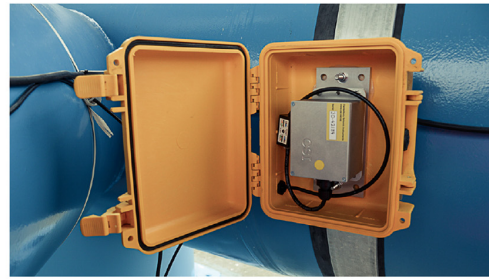
(b) CSI CUSP-3 accelerometer on truss. Opened protection box.
