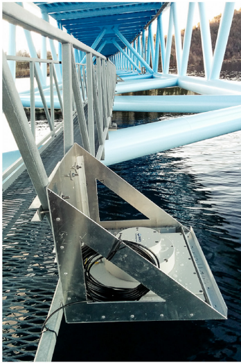
(c) Miros wave radar on walkway.
