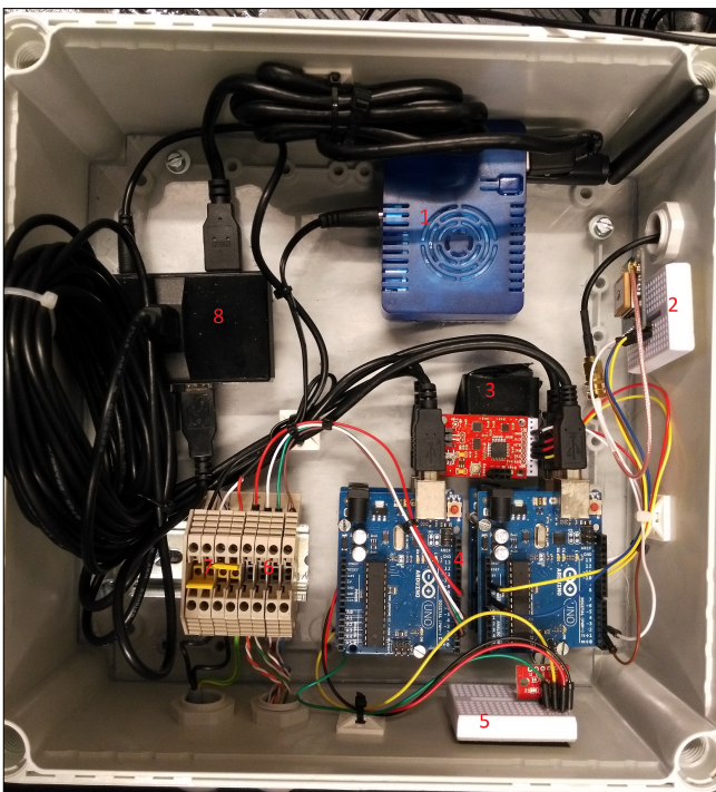
Fig. 8. Physical implementation of control system.
