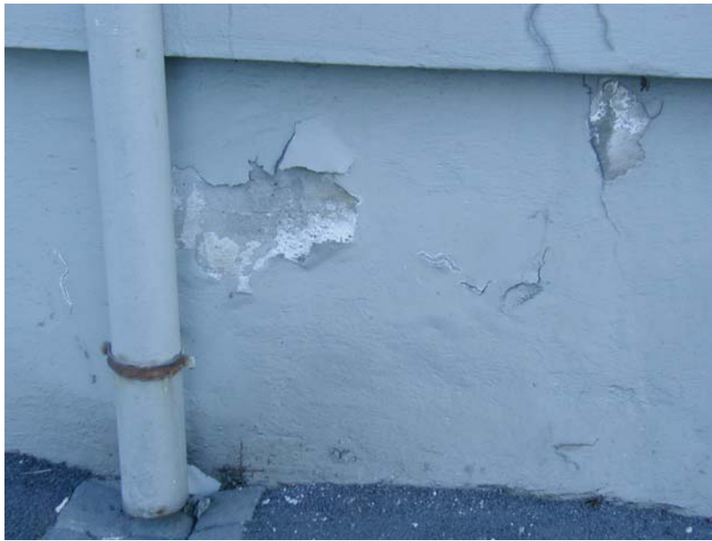
Figure 7. Flaking, PCB-containing paint from the surface of the indicated building in figure 6 (Photo: R.T.Ottesen).
