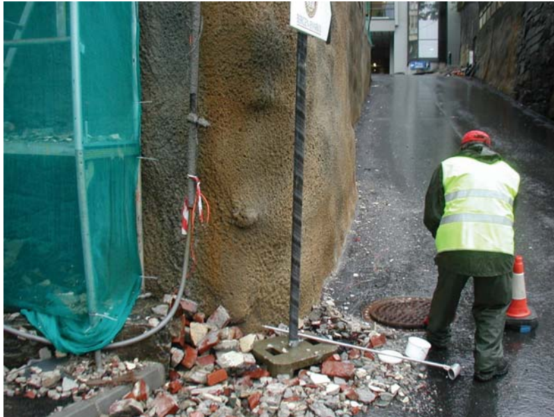
Figure 8. Renovation of contaminated building surfaces will enhance the mobilization of e.g. PCBs to the stormwater system (Photo: M.Jartun).
