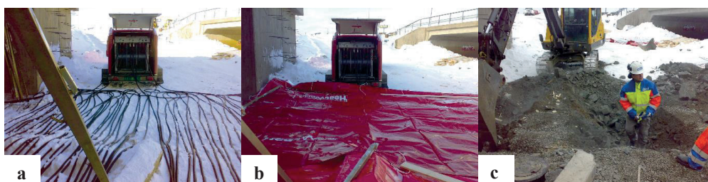
Figure 2. Hoses laid out on the area to be thawed, cured or protected from frost (a), insulation blankets covering the hoses to reduce convective heat loss (b), thawed ground ready for ground work (c). (Photos: Heatwork)
