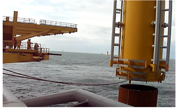
FIGURE 1: Mating phase between TP and Monopile using a heavy lift offshore mono-hull crane vessel
