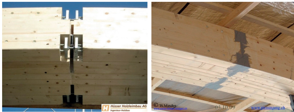
Figure 2.6 Example of application of glued-in rods in the apex of an arch bridge, Kirchenbrücke, 2009, Switzerland, [36]
