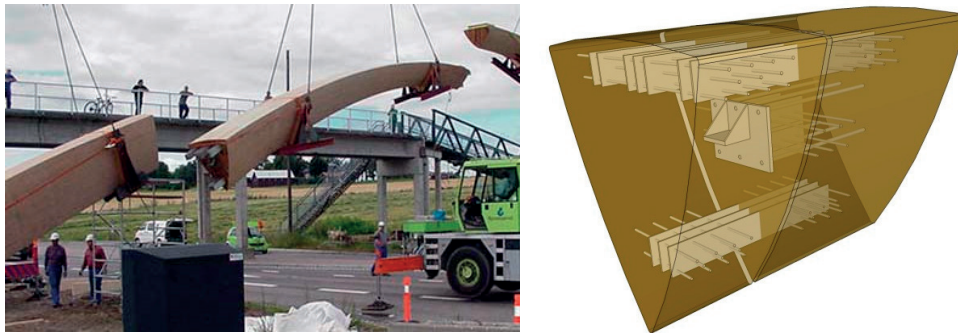
Figure 2.2 The Leonardo Footbridge (2001), Norway: the central arch under assembly (left), visualisation of the splice joint (right)
