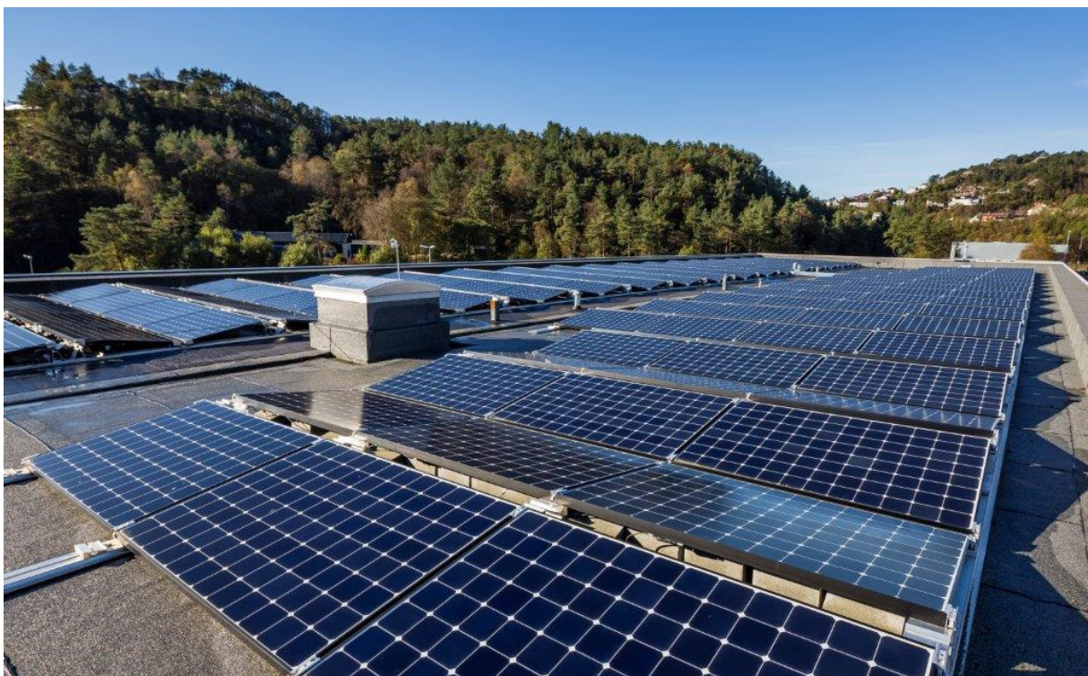
Figure 4.4 PV panels on the roof of Visund. Photo: Forsvarsbygg / Hundven-Clements Photography.
