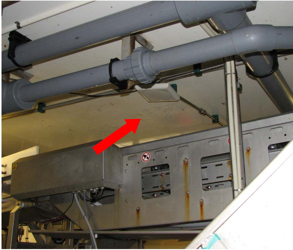
Figure 10: RFID antenna attached to factory ceiling, above conveyor belt to buffer tanks.
