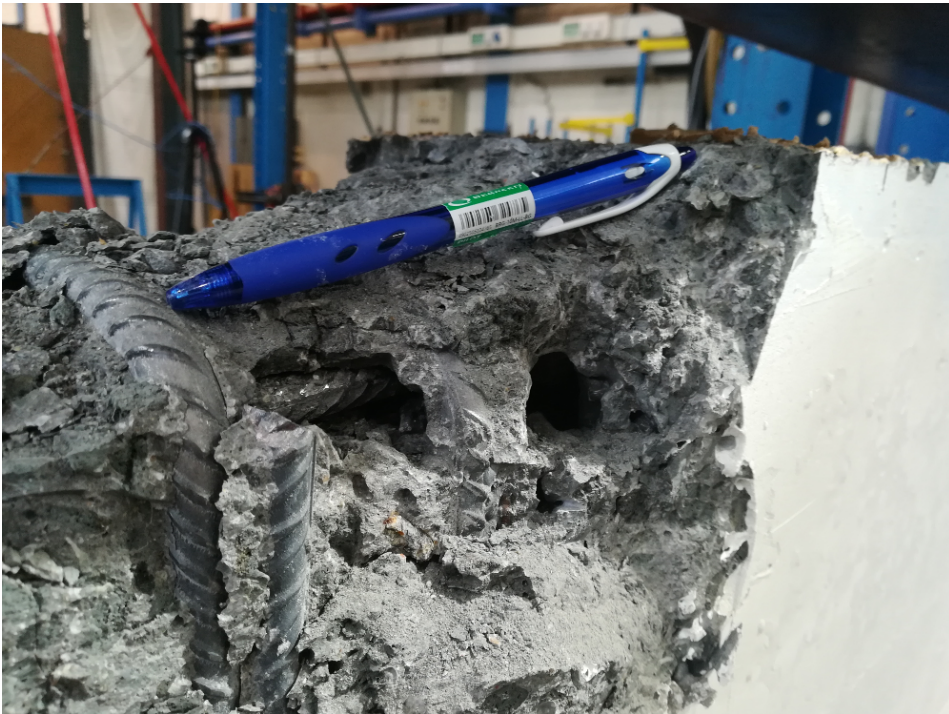
Figure 5.40: Visual pockets of air in the concrete
