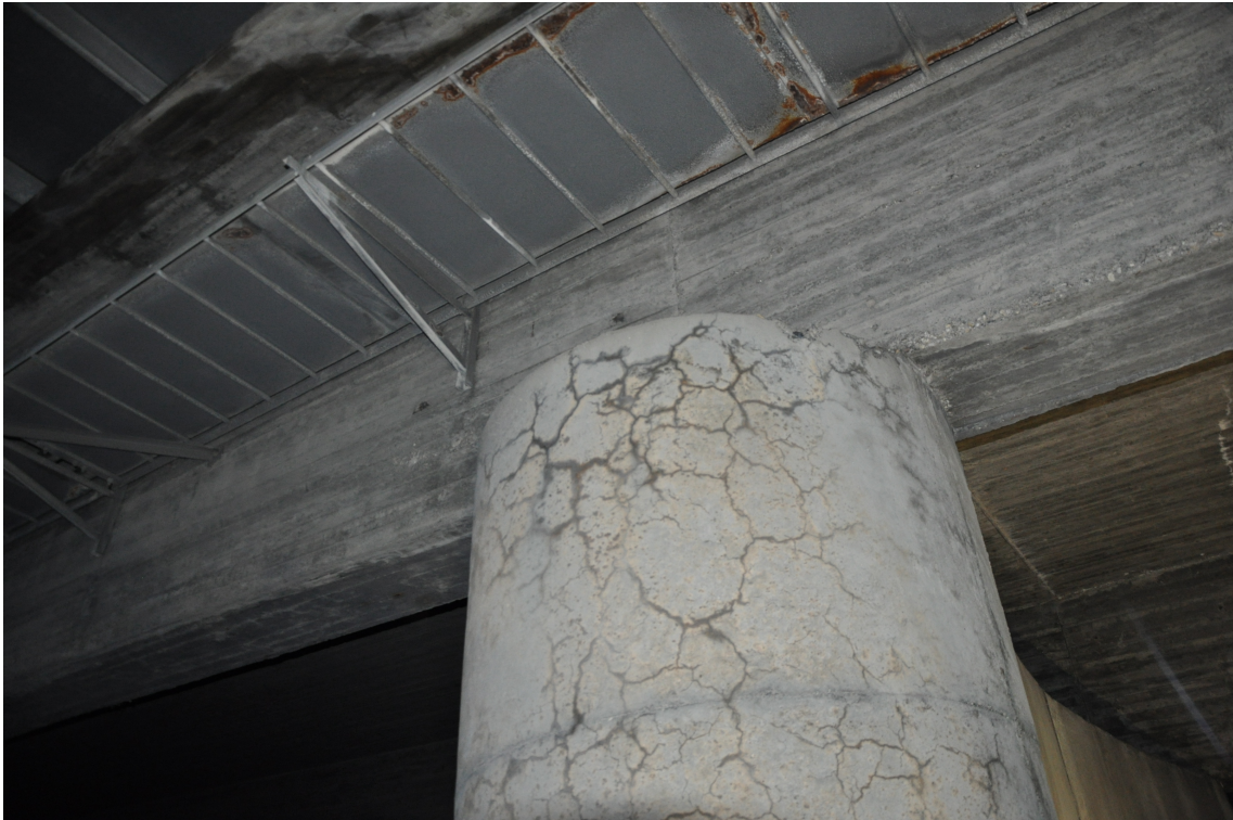
(a) Forsterket krakelering i toppen
