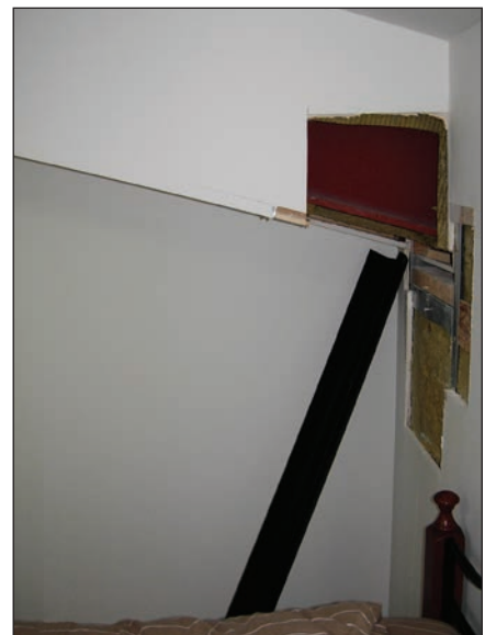
Photo 13: Ad hoc solution for temporarily coping with water ingress problem. It's almost like getting a Roman aquaduct in the bedroom.
