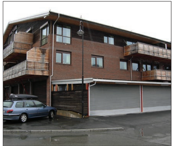
Photo 10: Combined business and apartment building experiencing water leakage problems from the roof, where investigations revealed that some of the leakage water was caused by snow and water inlet through the fresh air ventilation intakes.
