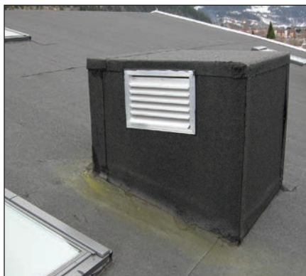
Photo 11: Apartment building air intake with no shielding.
