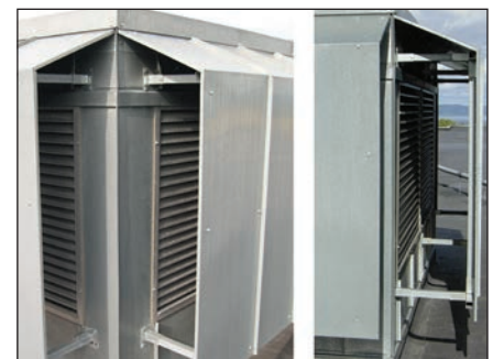
Photo 5: Shielded fresh air ventilation intakes. Note that it is also recommended to shield the open sides shown here, i.e., the only air intake is from under the shielding and upwards.
