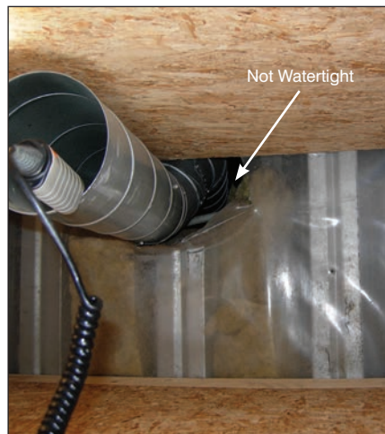
Photo 12: Inspection of an air intake revealed a non-watertight solution as a feedthrough pipe perforated the vapor barrier, allowing water to flow down into the building.
