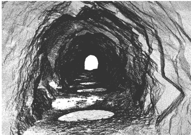
Figure 4: Typical tunnel view generated from a TLS point cloud. (Aberle, et al. , 2017)
