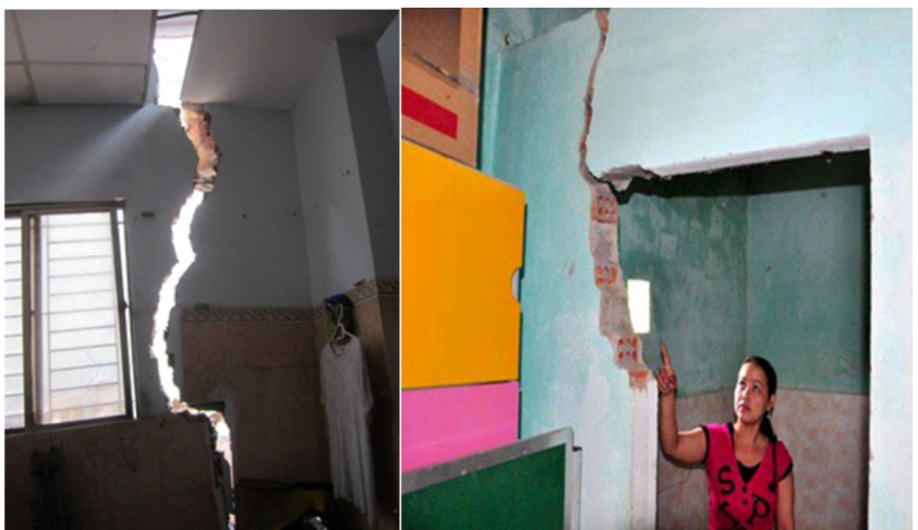
Figure 4: Damages in local homes, resulting from seismic activity at ST2 HPP.
