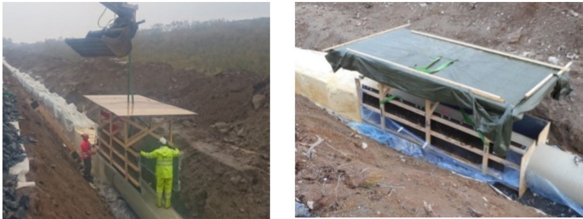
Figure 3: a) Formwork relocated with an excavator b) Formwork placed around the penstock
