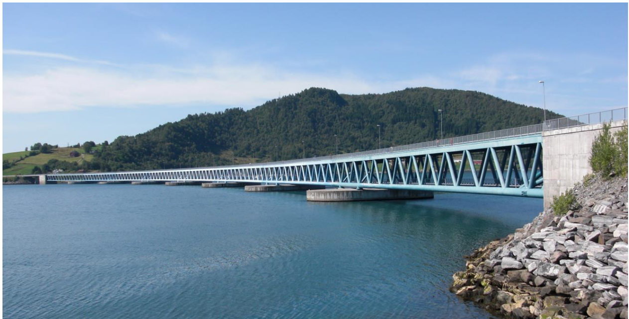
Figure 3: The Bergsøysundet bridge, with the steel superstructure clearly seen resting on the oval pontoons (Johs.holt, nd)
