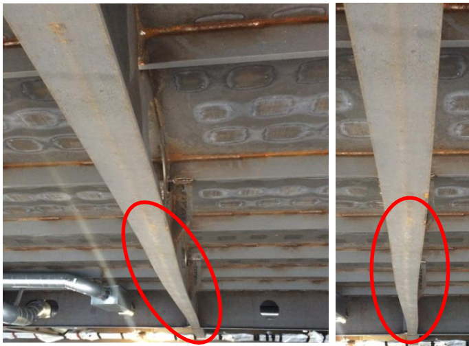
Figure 5.1: Production phase: defects in T-beams.
