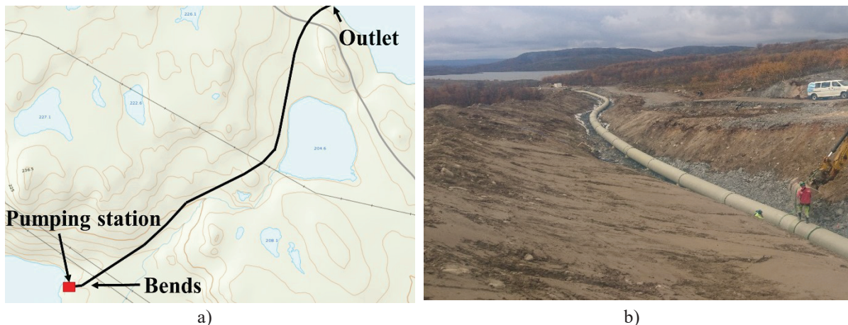
Figure 2: a) Map of the penstock alignment b) The penstock at Lille Måsevann
