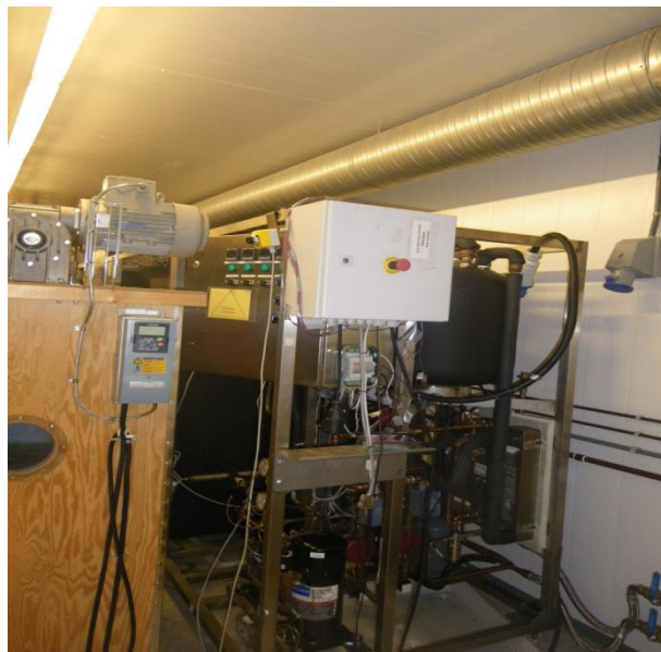
Figure 5.2 View of the control panel of the heat pump dryer
