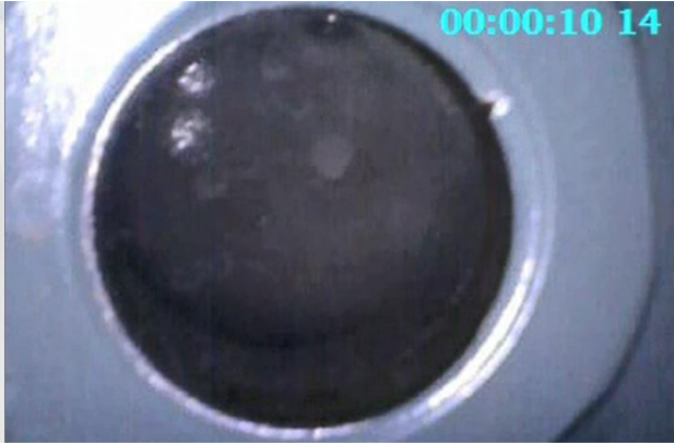
4. Superheat compressor suction 13K
