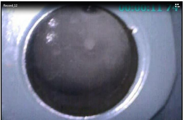
2. Superheat compressor suction 8K
