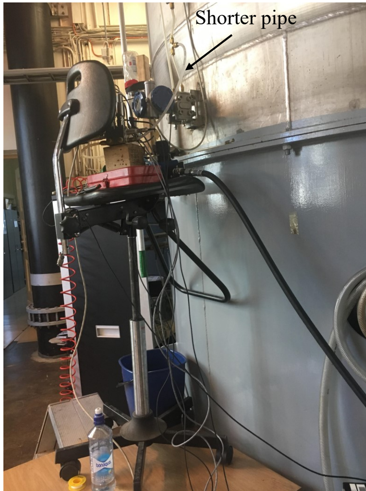
Figure 46 – Shorter pipe setup
