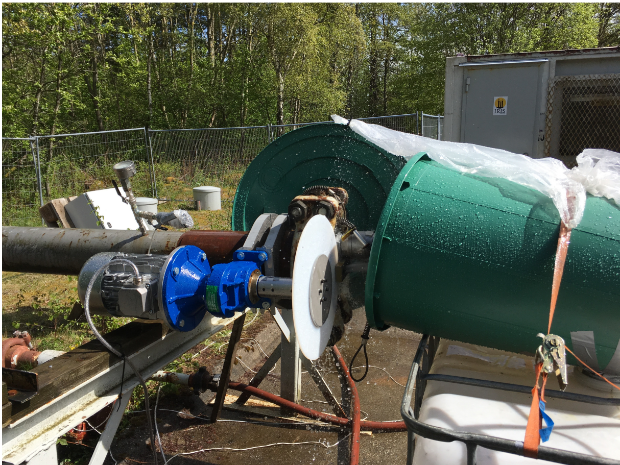
Figure B.7: Photograph of the collection bucket, a part of the water recycling system
