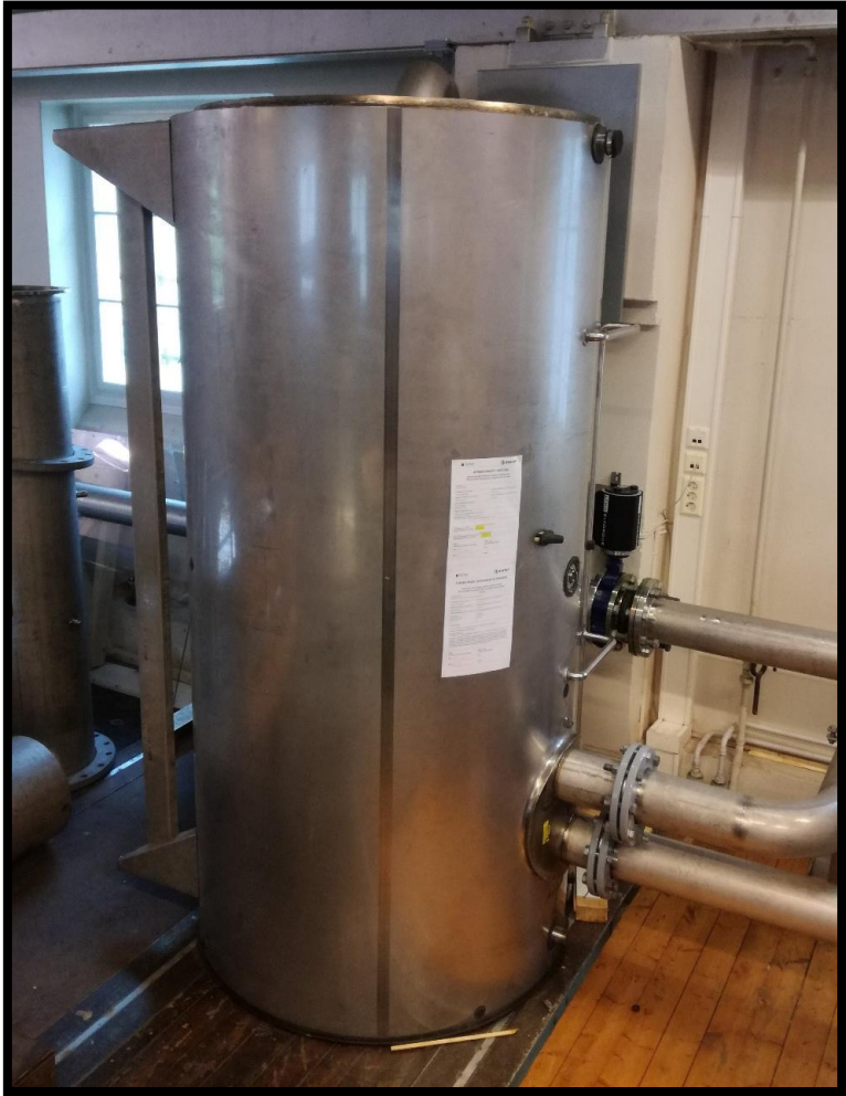
Figure F-3: Picture of the upper tank . Showing the outlet for the headrace and spillway
