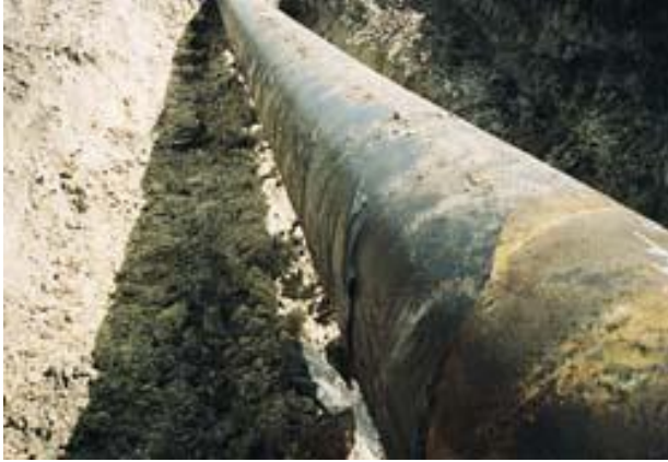
Fig. 15: Deteriorated coating on a 24-inch pipeline (Wilke et, al 1997)
