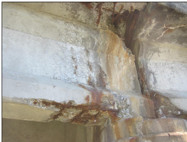
Figure 1-2: Deteriorated concrete beam due to reinforcement steel corrosion. The image is from [AlwaysCivil, 2011].
