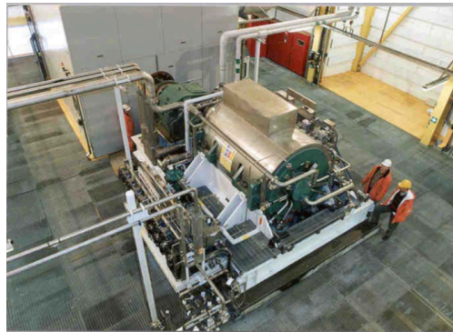
Figure 4: Compressors at Kollsnes [12]
