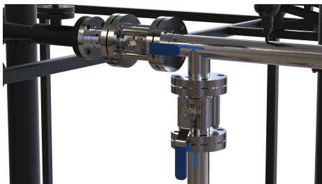
(a) Tee connection and 3-MV-101 and 3-MV-102 manual valves to divert inlet flow to GLCC or CFU respectively.
