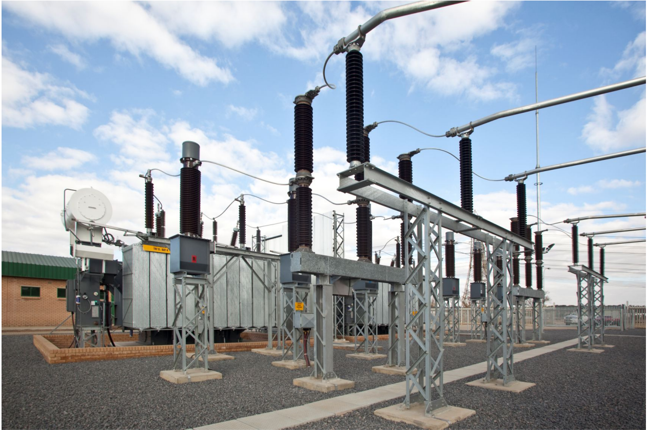
Figure 3.2: An illustrative substation switching yard. Bus bars of the three phases are shown in front, and they are connected through a CB and a measurement transformer to the power transformer in the back.
