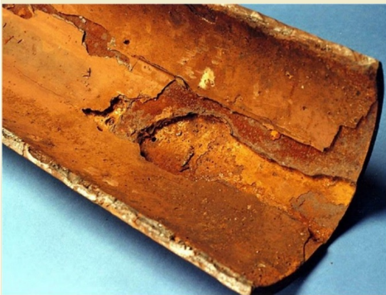
Figure 2.20: Internal corrosion of a pipe (Metropolitan Engineering Consulting and Forensics, 2016).
