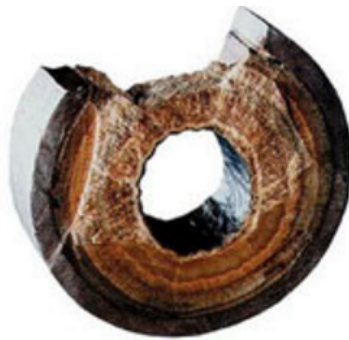
Figure 2.18: Scale in a pipe (Bai and Bai, 2010g).
