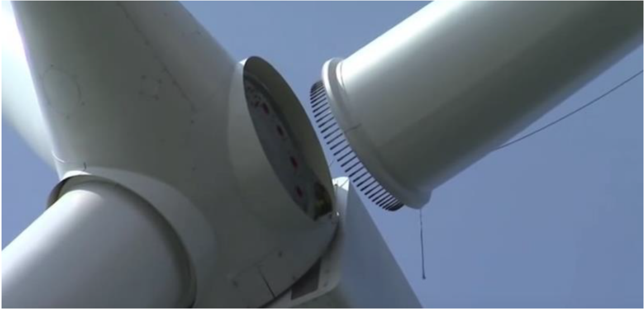
Figure 2.5: Mating of a blade on the rotor (from SeajacksUK Youtube Channel www.youtube.com/channel/UCpSMVnU3NyoTtQbhU73dU3w )
