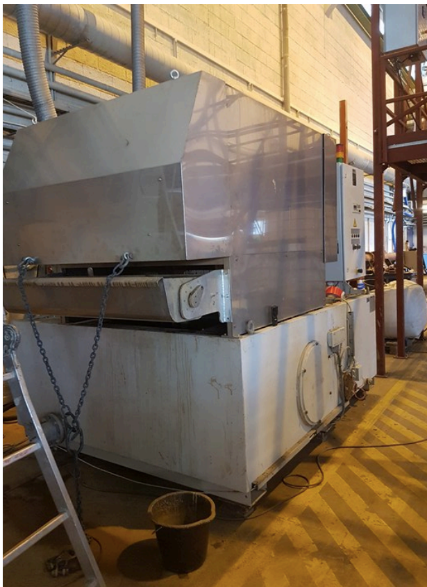
Figure 11 Sand filtration unit with mud tank and mixer
