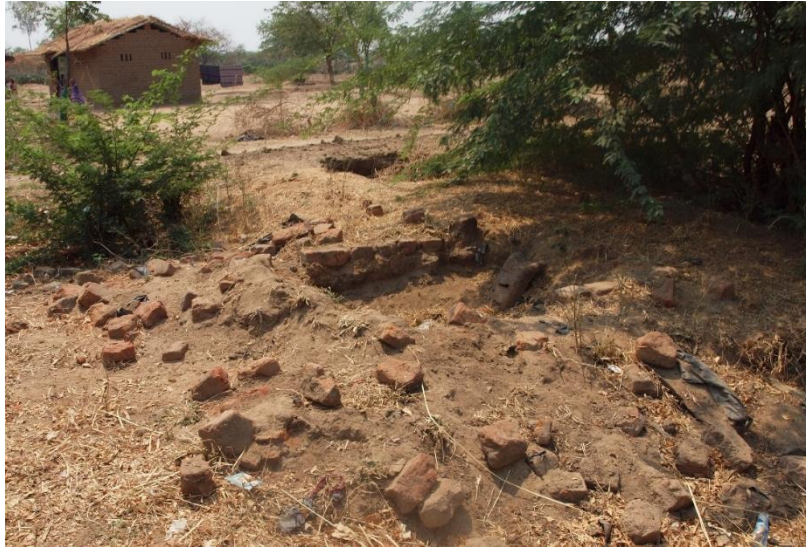
Figure 6.4: Photo showing a collapsed pit latrine in Alufandika Village, Nsanje (Photo: Author).
