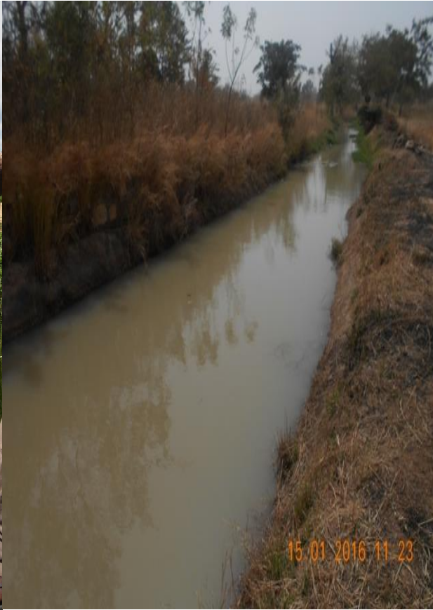
A Canal overgrown with weeds
