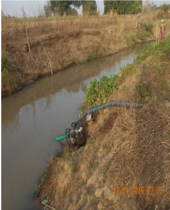
Water pumping machines
