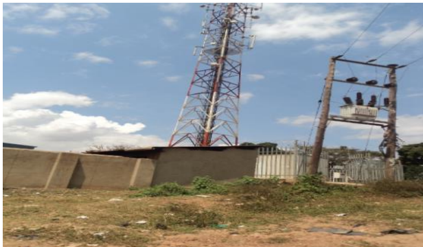
Figure 49: Power and Telecommunication installations within residential settlements
