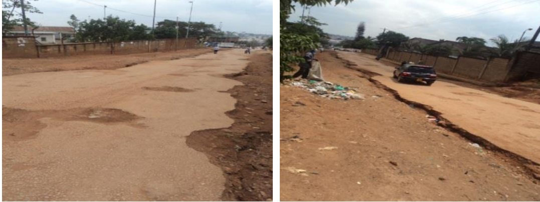
Figure 22: Some of seriously damaged roads
