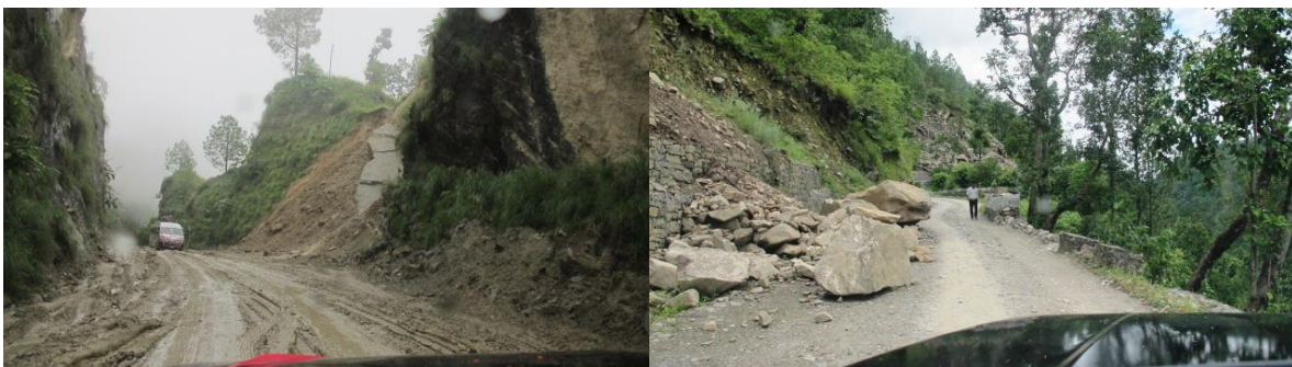
Figure 6-1 - Landslides and mudslides on the road from Surkhet to Dailekh (Holst 2012).
