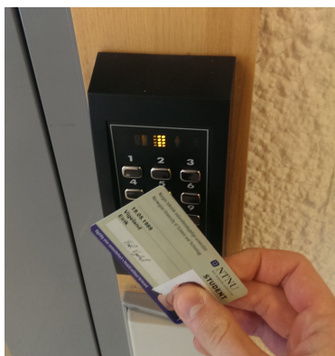
Figure 5.6: Common RFID access control.
