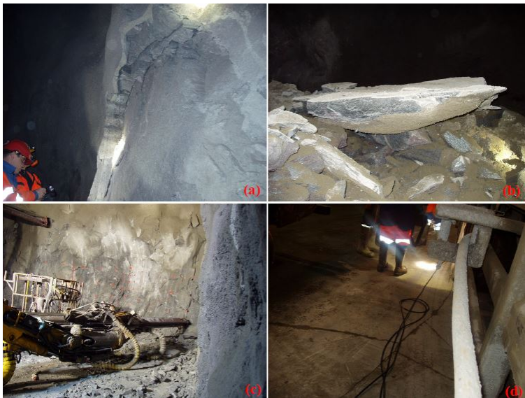
Figure 3.4: Stability issues during excavation of tunnels near the crusher hall in the mine. (a) Spalling in side wall. (b) Typical shape of spalling fallout. (c) Rock burst at front face. (d) Cracks in floor resulting from heaving (Trinh et al., 2010).
