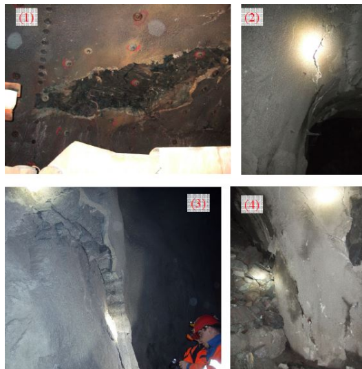
Figure 3.6: Failure of shotcrete in different parts of cross section (Trinh et al., 2010).
