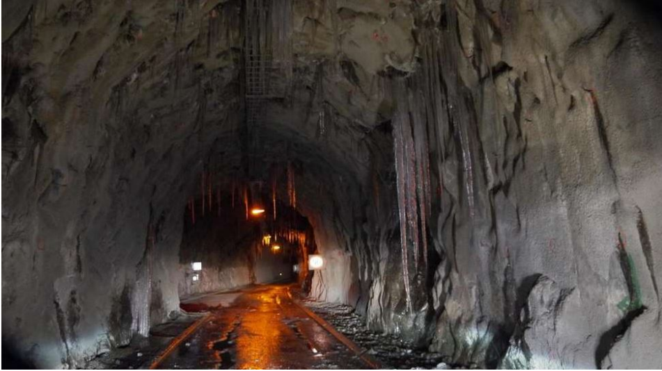
Figure 2.7: Illustrative photo from a road tunnel ruined by ice, near Øksfjord in Finnmark. The Øksfjord-tunnel is deemed the "tunnel of shame" by the director of the Norwegian newspaper Altaposten . ( Altaposten [Online], 2013).
