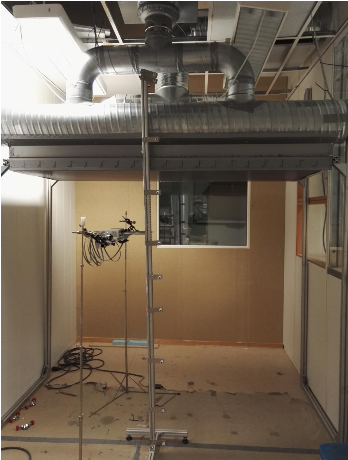
Figure D.4 - Placement of the air distribution measurement equipment
