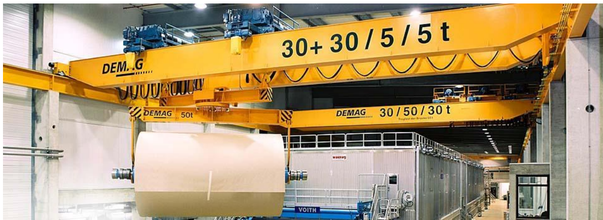
Figure 7 Demag process crane handling paper rolls (Demagcranes, 2017)
