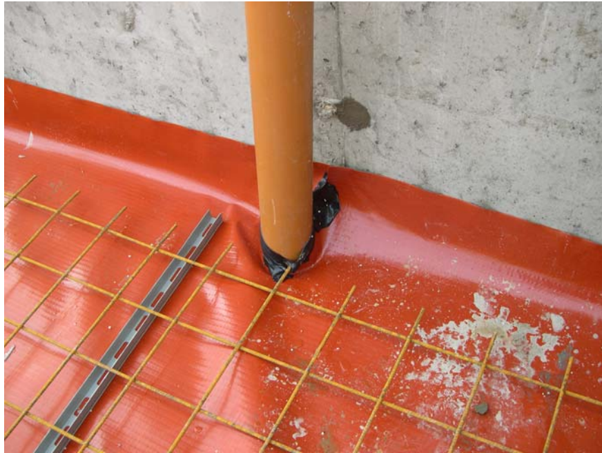
Fig.7. Air leakage through or in connection with the radon barrier might be caused by several factors. The photo above depicts a reinforcement bar with support which represents a risk for perforation of the radon barrier. To ensure satisfactory airtightness around feed-through pipes might be difficult, especially close to walls or other obstructions. In addition, satisfactory airtightness must also be ensured towards the concrete wall.
