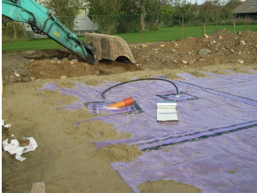
Fig.3. By placement of radon barriers it is essential to ensure satisfactory airtightness in joints and various feed-throughs.
