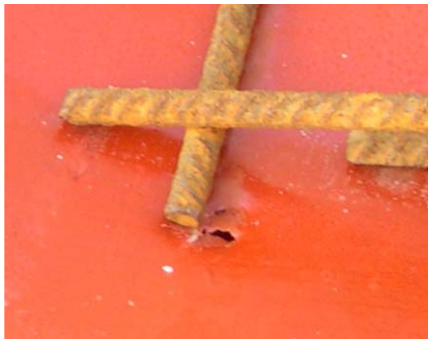
Fig.8. Care has to be taken in order to avoid any perforations in the radon barrier. This example depicts a reinforcement bar which has perforated the radon barrier.
