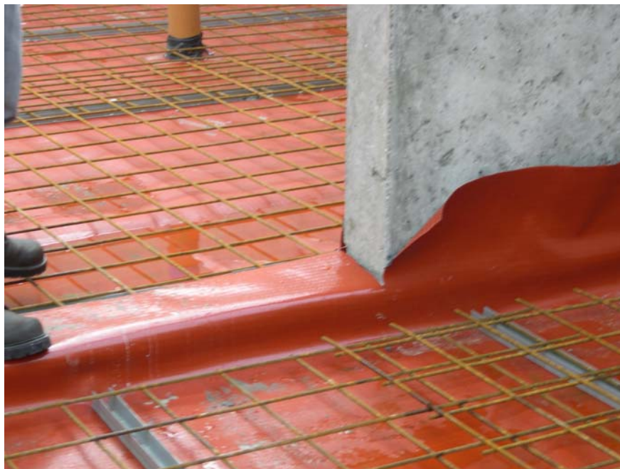
Fig.10. Various junctions, corners and turn-ups represent areas where proper care has to be taken in order to obtain satisfactory airtightness. Care has to be taken during cutting of the radon barrier.
