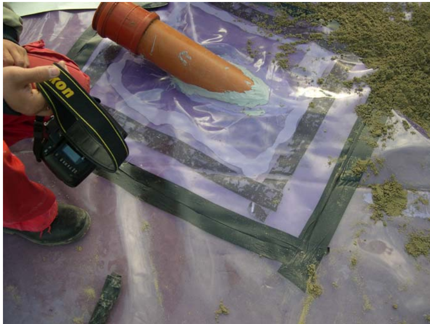
Fig.4. Trying to ensure satisfactory airtightness in a radon barrier at a feed-through pipe applying a sealant. Close-up from fig.3.
