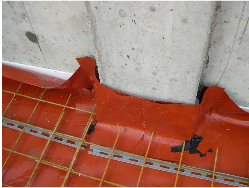
Fig.9. Outer and inner wall corners represent another area where proper care has to be taken in order to obtain satisfactory airtightness.
