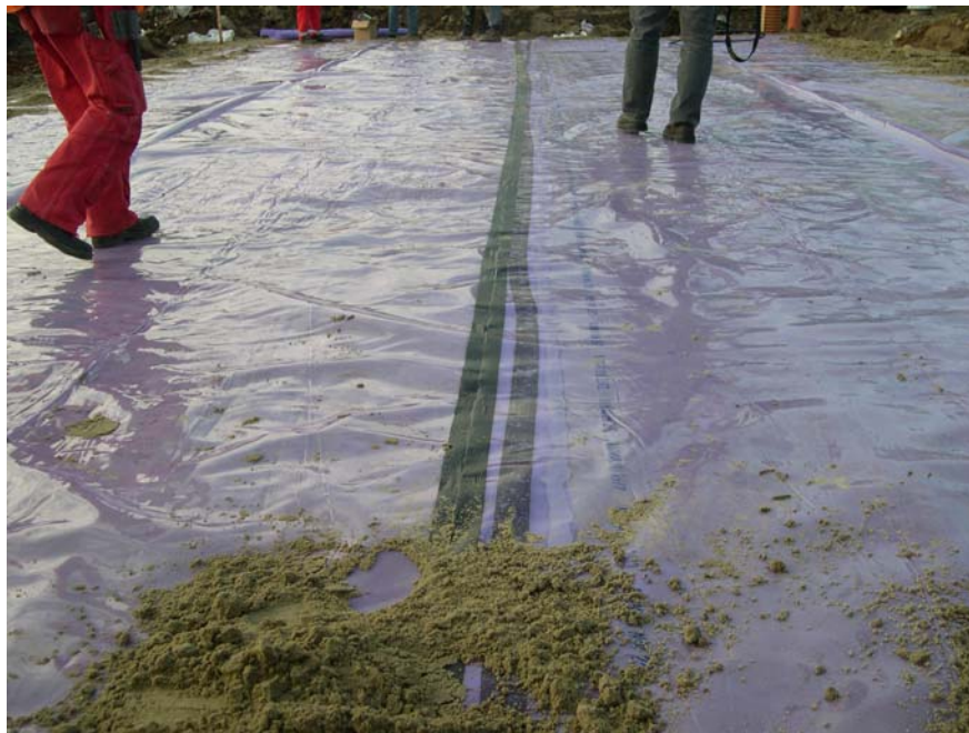
Fig.6. Joints have to be satisfactory airtight and care has to be taken when people are walking on the radon barrier before covering, in order to avoid any perforations.
