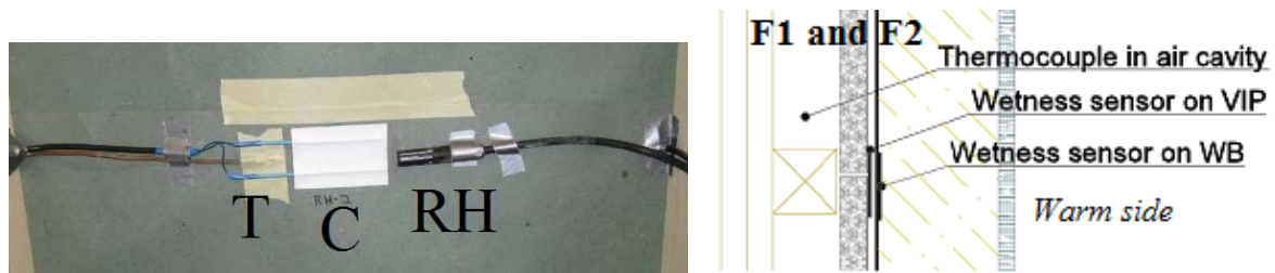
Figure 7. Left photo depicts the thermocouple (T), wetness sensor (C), and RH air sensor (RH) as installed on the wind barrier before the mineral wool was added. Right drawing shows a cross-section of F1 and F2 with a wetness sensor both on the wind barrier and on the joint between two VIPs at the middle of the fields. The thermocouple in the air cavity is also shown, while other sensors on the wind barrier (WB) are not depicted.
