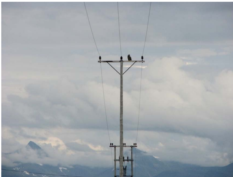
Figure 9. Eagle owl perching on the crossarm of a 22kV pole (no 148). Pole no 149 with pole mounted transformer in the background where bones of one dead eagle owl was found in July 2008. Two dead eagle owls were recorded beneath the same pole in spring 2005. Photo: Jan Ove Gjershaug.
