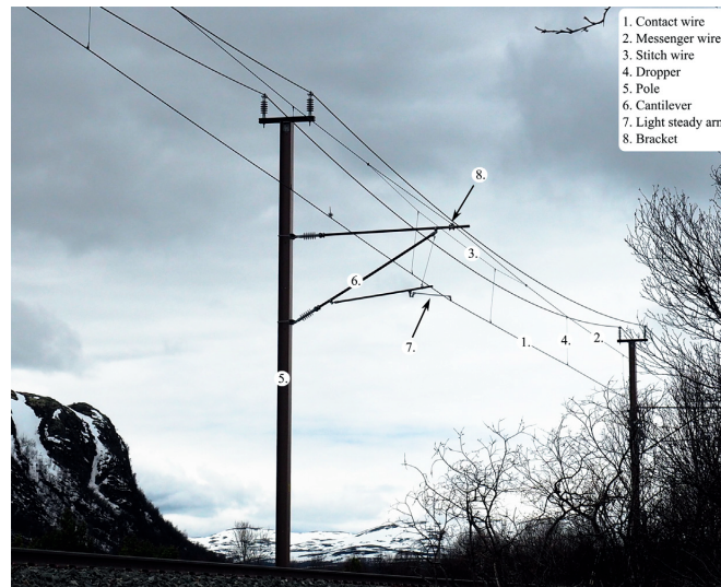
Fig. 2. Main structural components of a railway catenary system. Photo: Petter Návik/NTNU.
