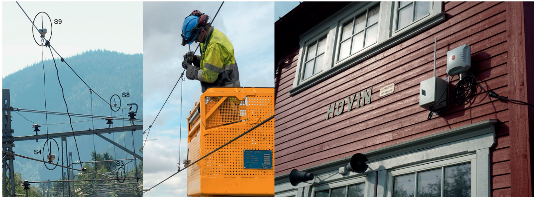
Fig. 6. Mounted monitoring system at the Hovin station: left—sensors; middle—mounting of a sensor; right—master unit and wireless wide-area network antenna. Photo: NTNU/Petter N avik.
