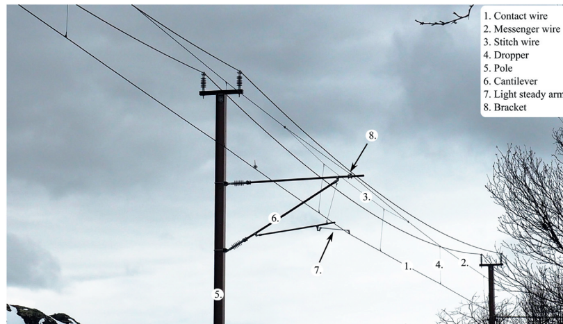
Fig. 3. Presentation of important structural components of railway catenary systems. Photo: NTNU/Petter Návík [10].
