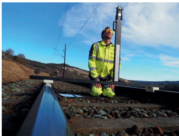
Figure 10. Measurement of contact wire height and stagger using a laser. Photograph: NTNU/Petter N avik
