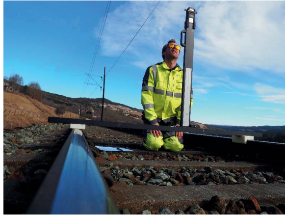
Figure 5. Measuring contact wire heights on site
