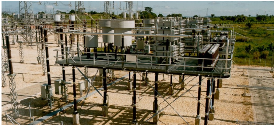
Figure 2.7: TCSC system delivered by ABB in Imperatriz, Brazil.
