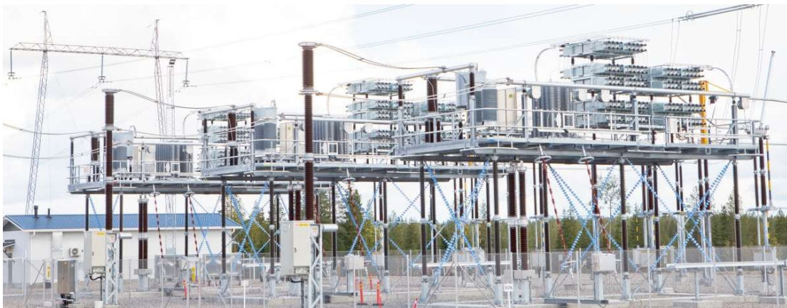
Figure 2.3: Fixed series capacitor system delivered by ABB in Asmunti, Finland
