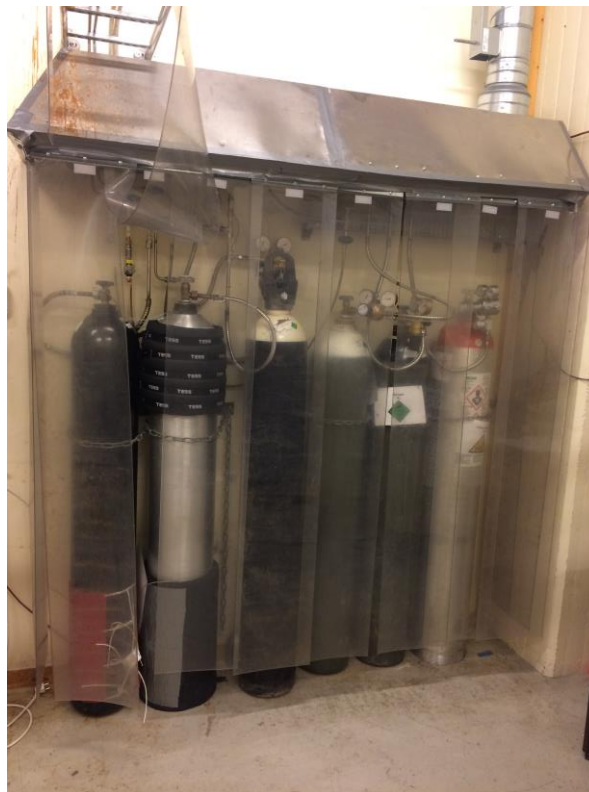
Figure 7: Gas Bottles Inside the Gas Mixing Room
