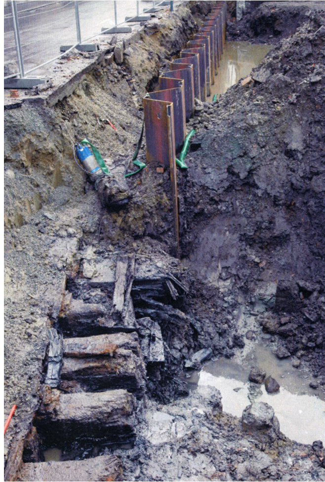
Figure 7: The exposed timber from the ship at Nedre Bakklandet in Trondheim. Shows the steel sheet pile wall. Photo: Fredrik Skoglund.
