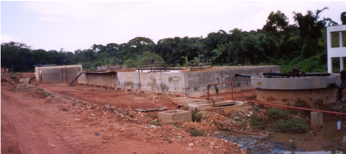
Figure 6: This picture shows the leachate treatment plant at Mpererwe landfill.
