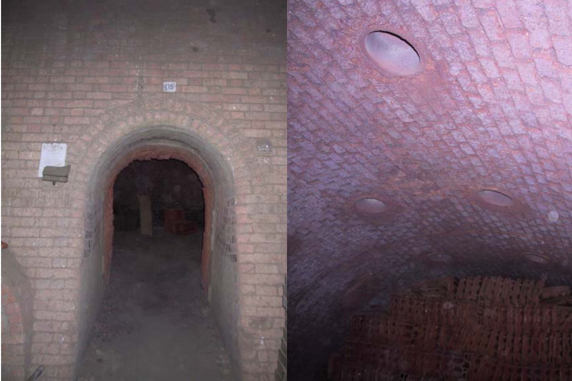
Figure 11: The entrance to one of the chambers in the Hoffmann kiln at Uganda Clays can be seen to the left. The right picture is showing the wholes in the ceiling of the kiln used to feed coffee husks into the kiln.
