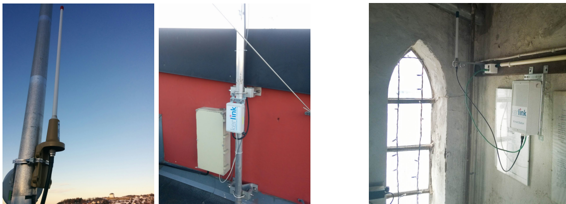
Figure 5: Deployment of LoRaWAN antenna gateway outdoors on the roof of the Student Society building in Trondheim (left) and elevated indoors in a clock tower in Vejle (right).
